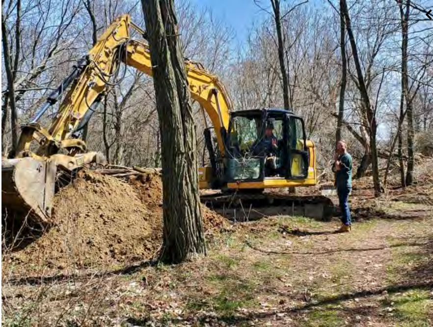
Property owner Ron Clapp is standing near an excavator on his Carleton Island property. Contributed.
