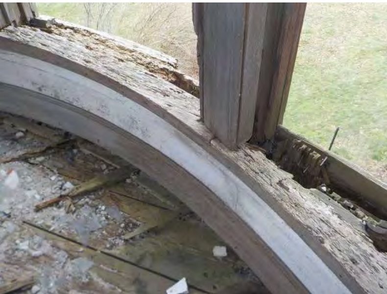
101 - Second Floor - Deteriorated exterior wall 3.jpg
