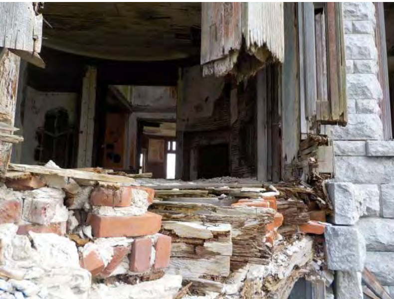
045 - Exterior masonry - Deterioration of top of wall 3.jpg
