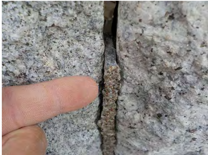
054 - Masonry - Condition of mortar joints 9.jpg
