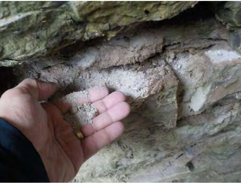
049 - Masonry - Condition of mortar joints 4.jpg
