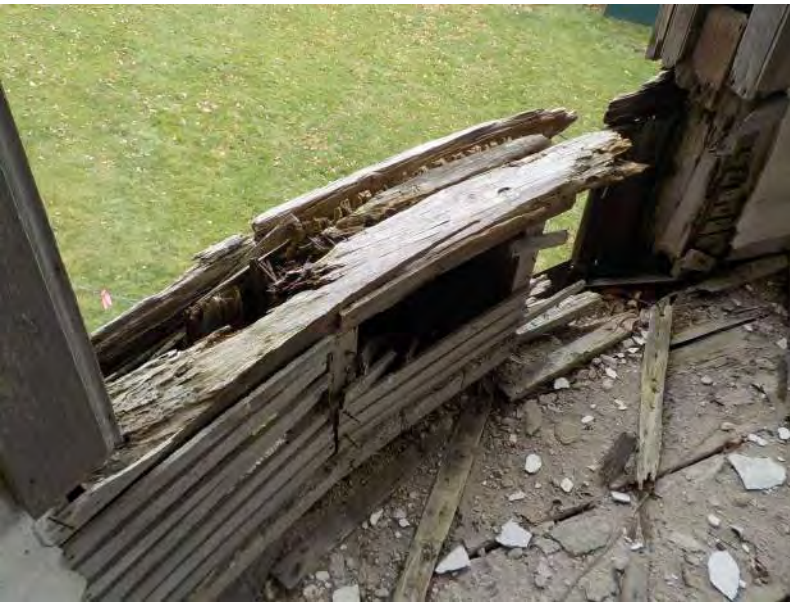
099 - Second Floor - Deteriorated exterior wall 1.jpg
