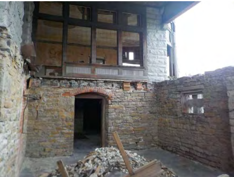
135 - Basement - Missing first floor at south corner.jpg
