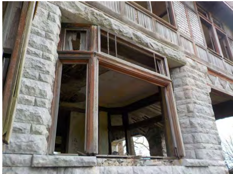
040 - Exterior masonry - Deteriorated support at window 1.jpg
