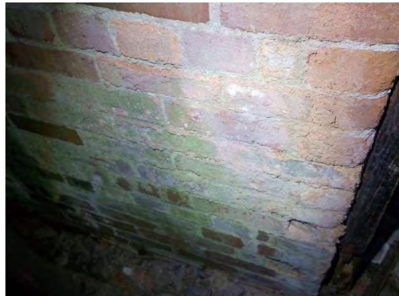
144 - Basement - Exfoliated brick wall near staircase.jpg
