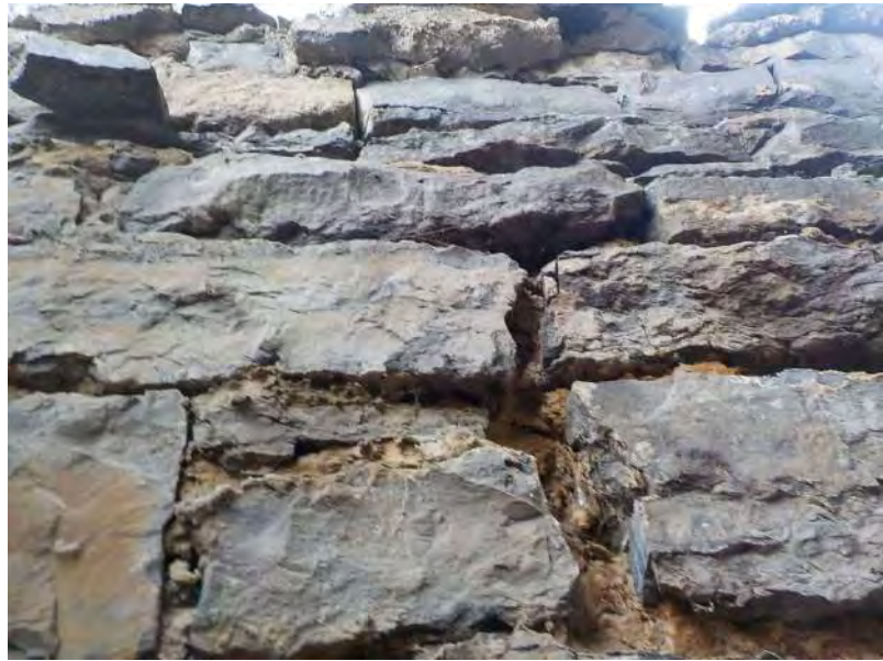
050 - Masonry - Condition of mortar joints 5.jpg
