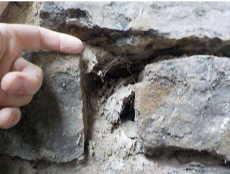
047 - Masonry - Condition of mortar joints 2.jpg
