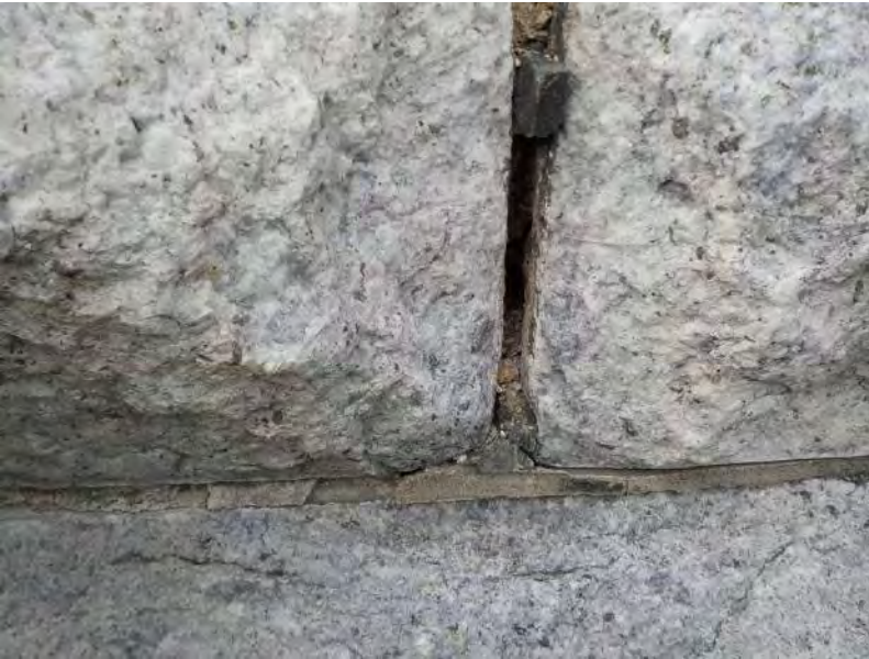
051 - Masonry - Condition of mortar joints 6.jpg
