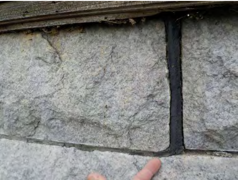
053 - Masonry - Condition of mortar joints 8.jpg
