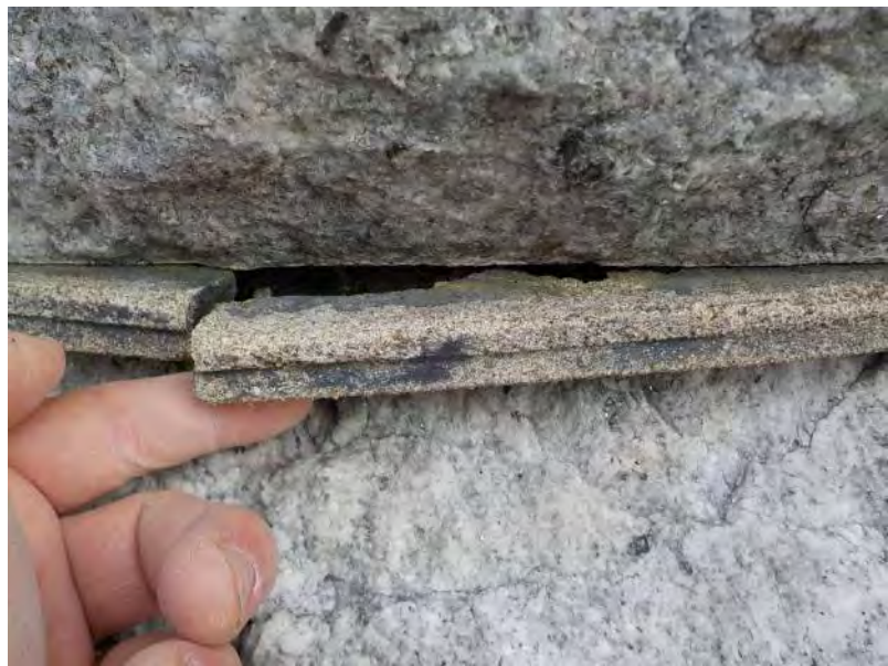
056 - Masonry - Condition of mortar joints 11.jpg
