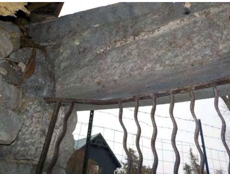
155 - Basement - Stone lintel with compromised end.jpg
