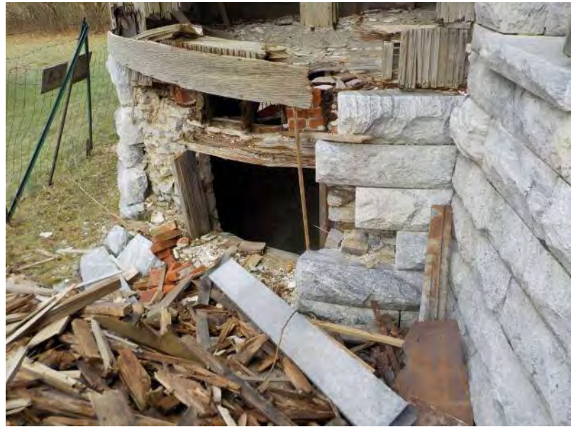
044 - Exterior masonry - Deterioration of top of wall 2.jpg
