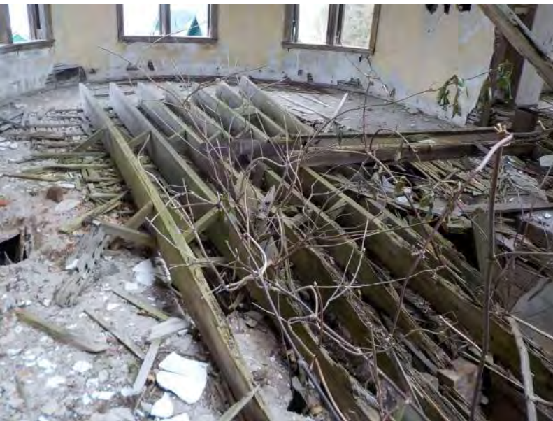
087 -Third Floor-Floor with fallen fourth floor framing1.jpg
