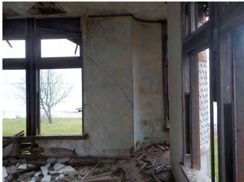
102 - Second Floor - Diagonal cracking in SW wall.jpg
