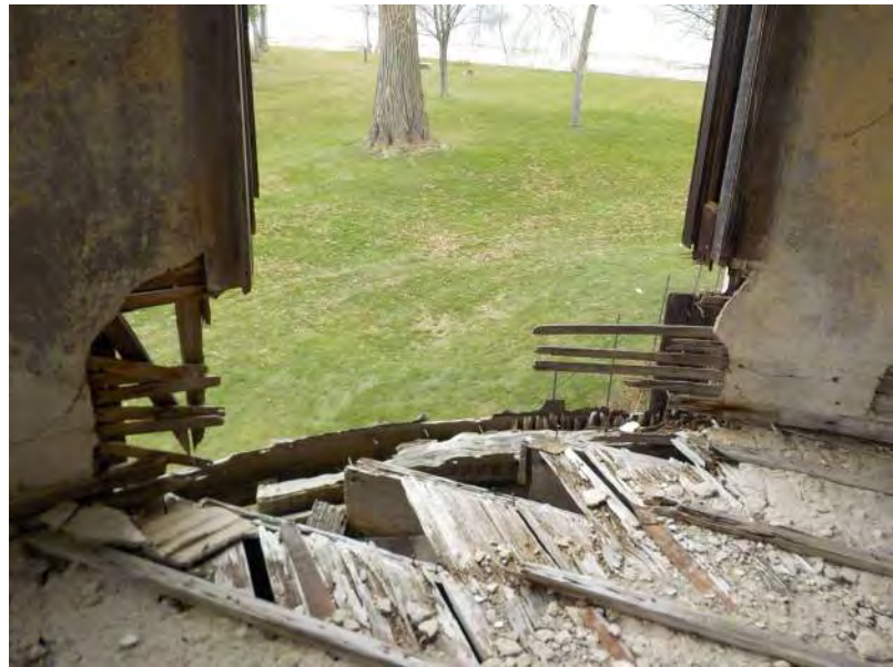
100 - Second Floor - Deteriorated exterior wall 2.jpg
