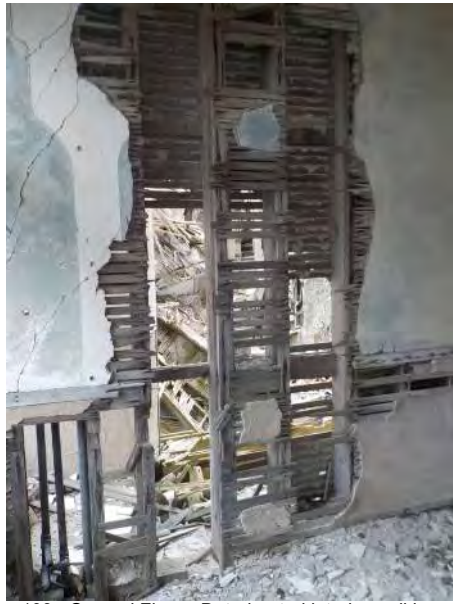
103 - Second Floor - Deteriorated interior wall.jpg
