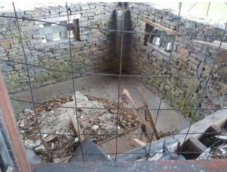
137 - Basement - Overview through missing floor at S corner.jpg
