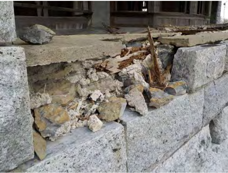
043 - Exterior masonry - Deterioration of top of wall 1.jpg
