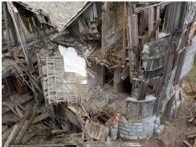
076 - Northeast Area - Collapsed section.jpg
