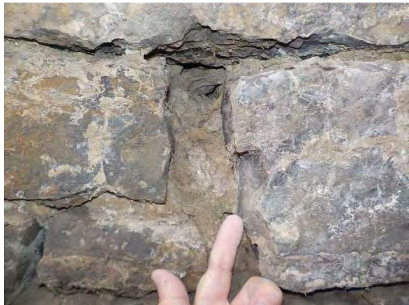
048 - Masonry - Condition of mortar joints 3.jpg
