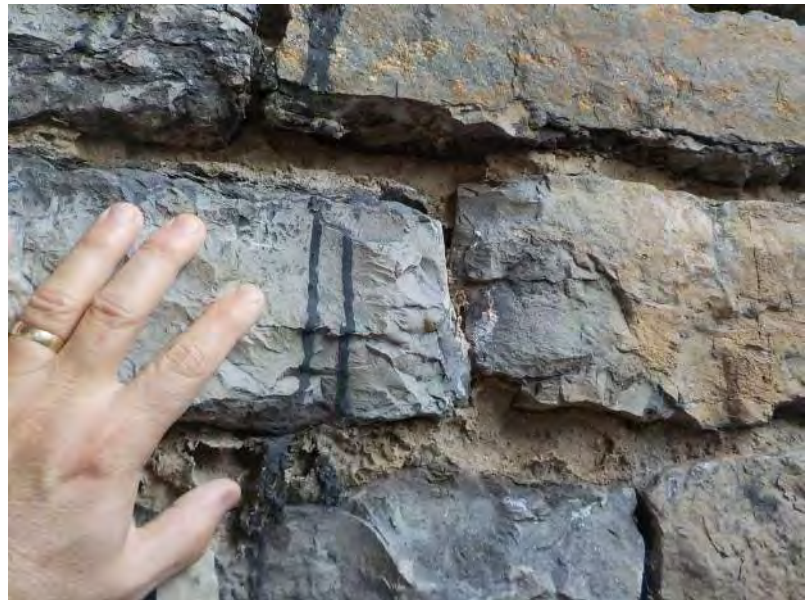
046 - Masonry - Condition of mortar joints 1.jpg
