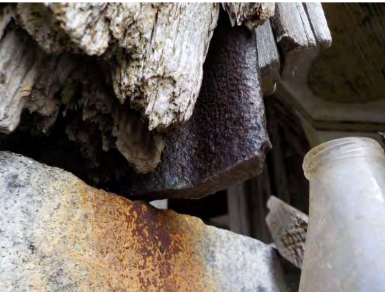
041 - Exterior masonry - Deteriorated support at window 2.jpg
