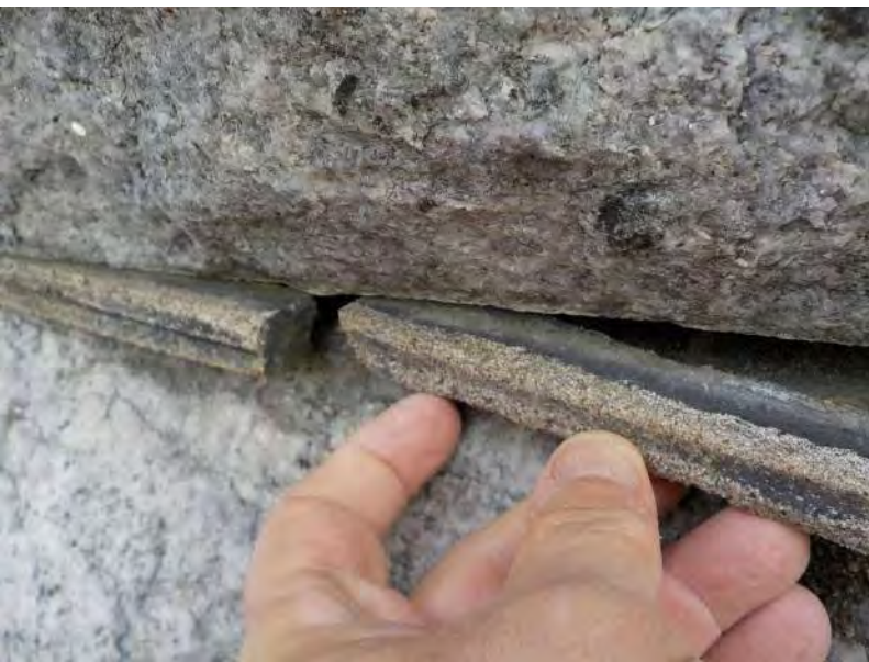
055 - Masonry - Condition of mortar joints 10.jpg
