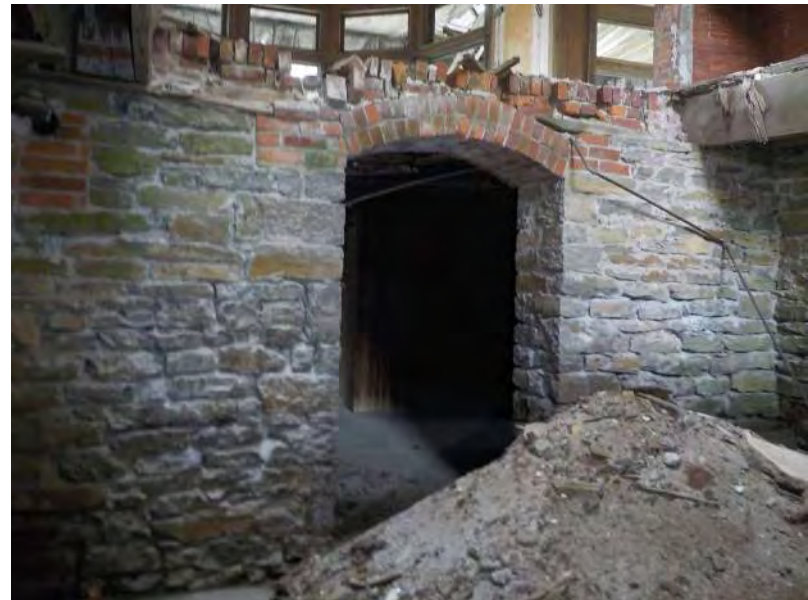
136 -Basement wall & opening at missing floor at S corner.jpg
