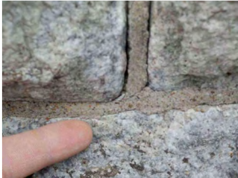
052 - Masonry - Condition of mortar joints 7.jpg
