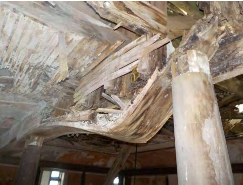
097 - Distressed 3rd floor beam from 2nd floor.jpg
