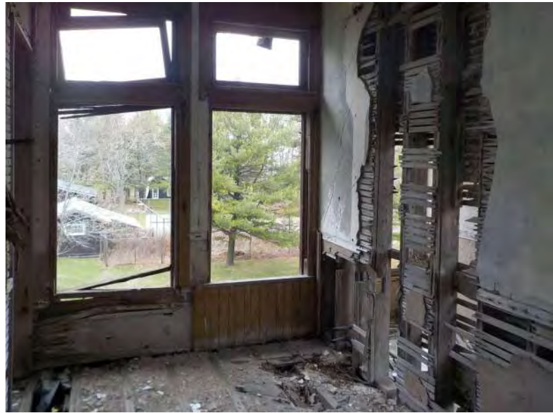
098 - Second floor deteriorated walls.jpg
